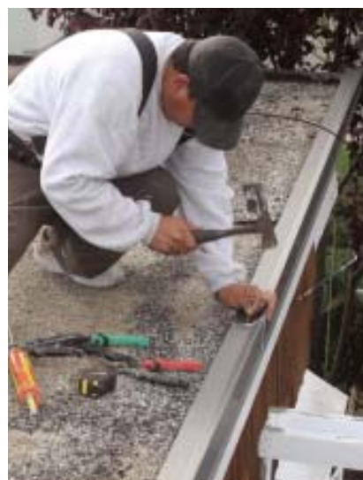
Figure 3. Before SPF is applied, the existing gravel stop is removed (above) and replaced with a new stop designed for foam. The crew uses polyurethane sealant and at least two nails at every lap (right) to prevent the joints from flexing and cracking. Next, the stop is nailed 9 inches o.c. to the edge of the roof.
