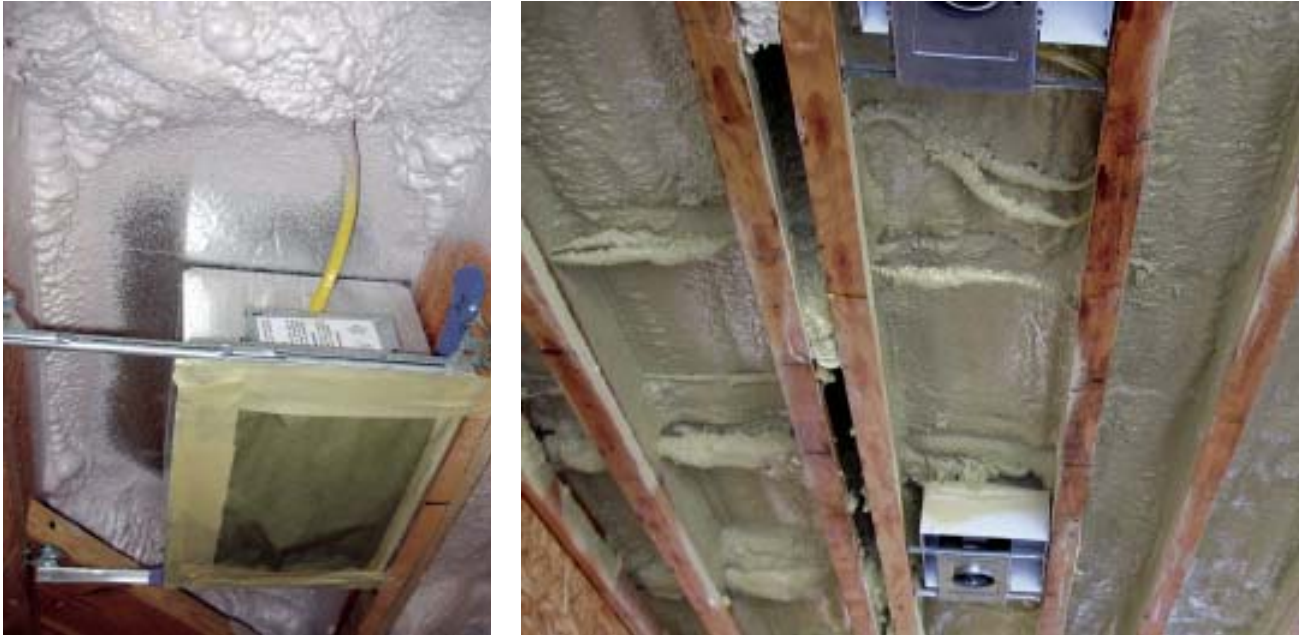
Figure 7. Code requires that a space be left between can lights — even IC-rated cans — and spray foam insulation. In shallow bays, the author’s crew installs foil-faced rigid foam above fixtures and creates a seal by lapping the spray foam onto it (left). An alternate method, which may soon be required in California, is to isolate fixtures from the foam by installing them in metal boxes (right).
